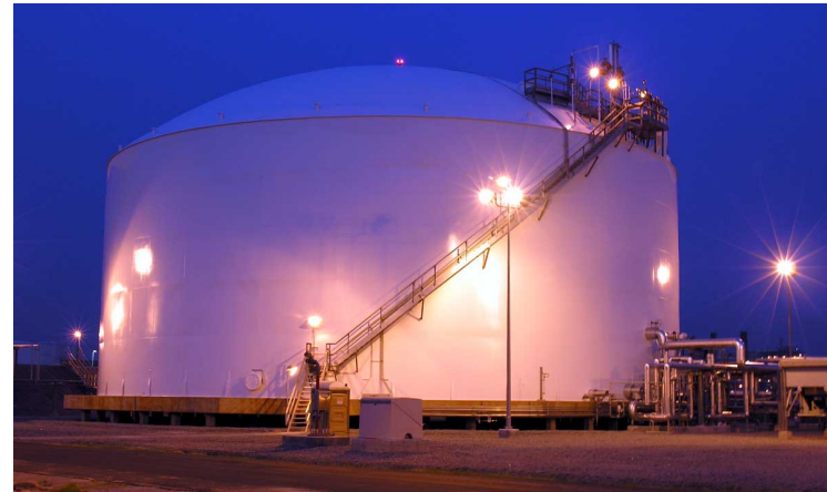
LPG/LNG Storage & Facilities
