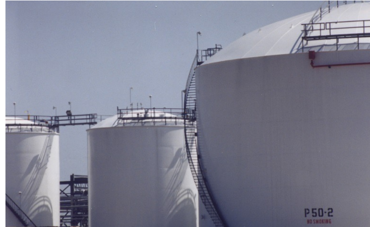
Chemical Storage Tanks
