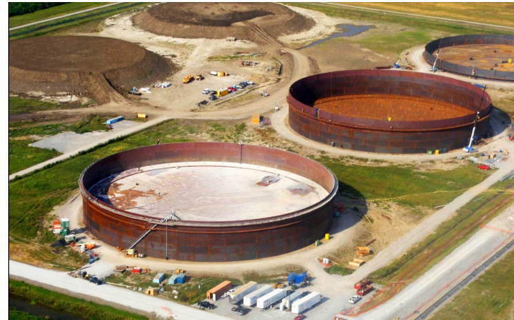
(6) 310' Dia. EFR API-650 Tanks
